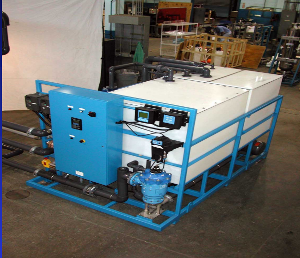
New Control Skid Assembly
