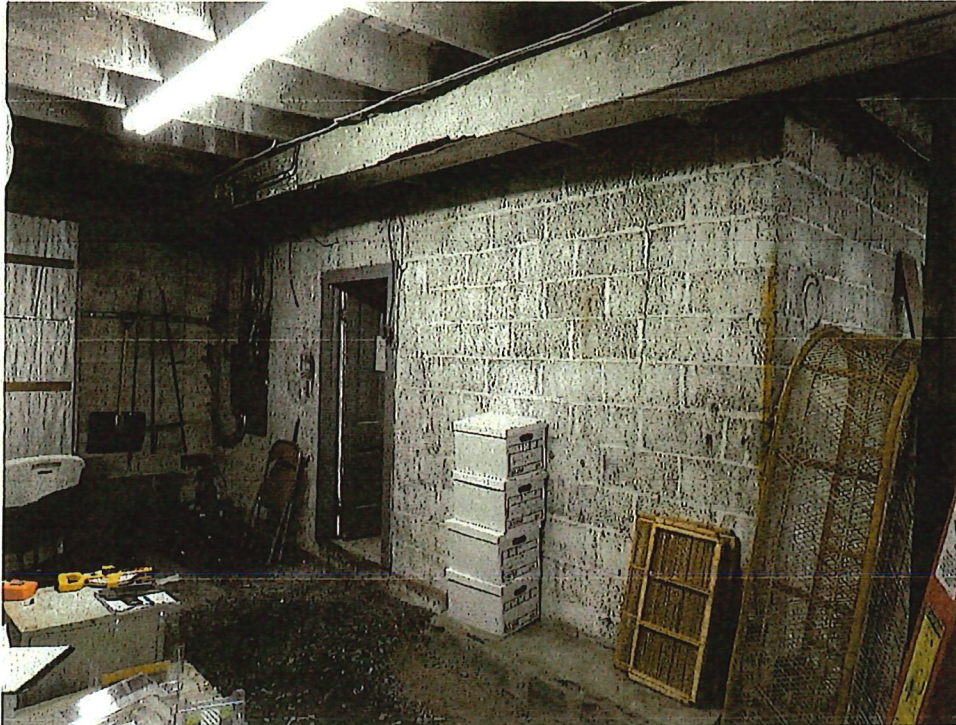
Figure 7 - Interior CMU partition, settlement cracking both sides of corner.
